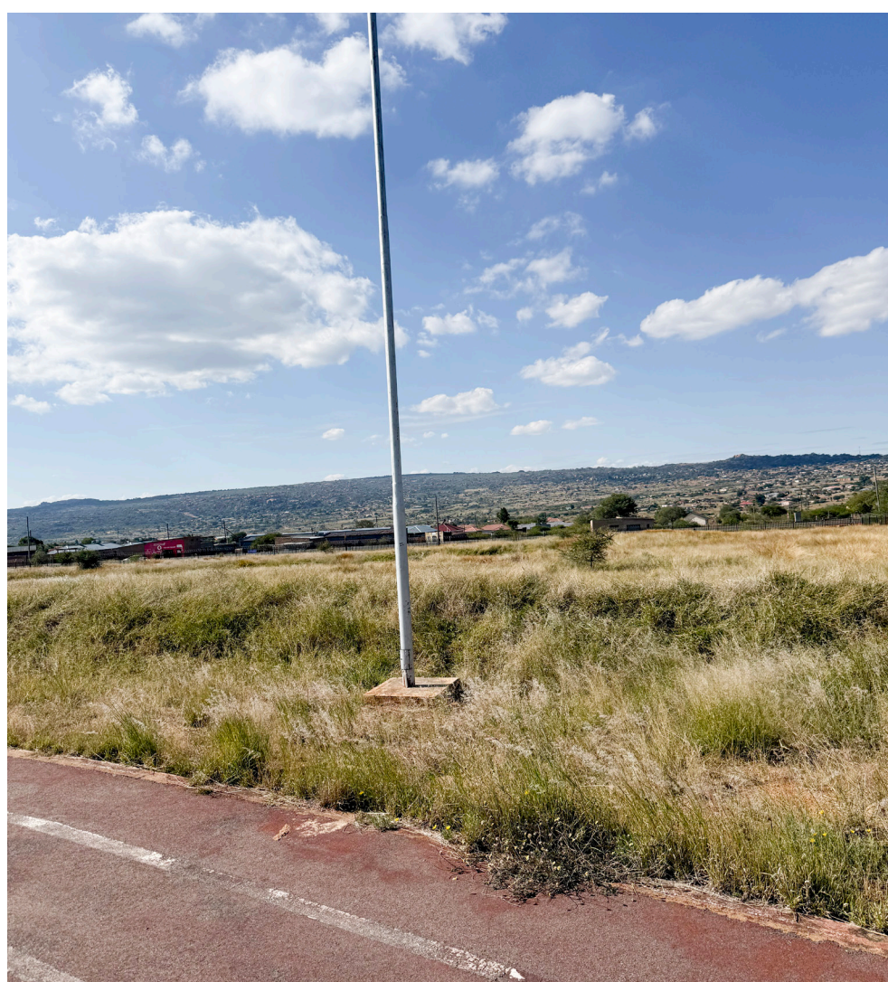
High-mast lights are failing the community
